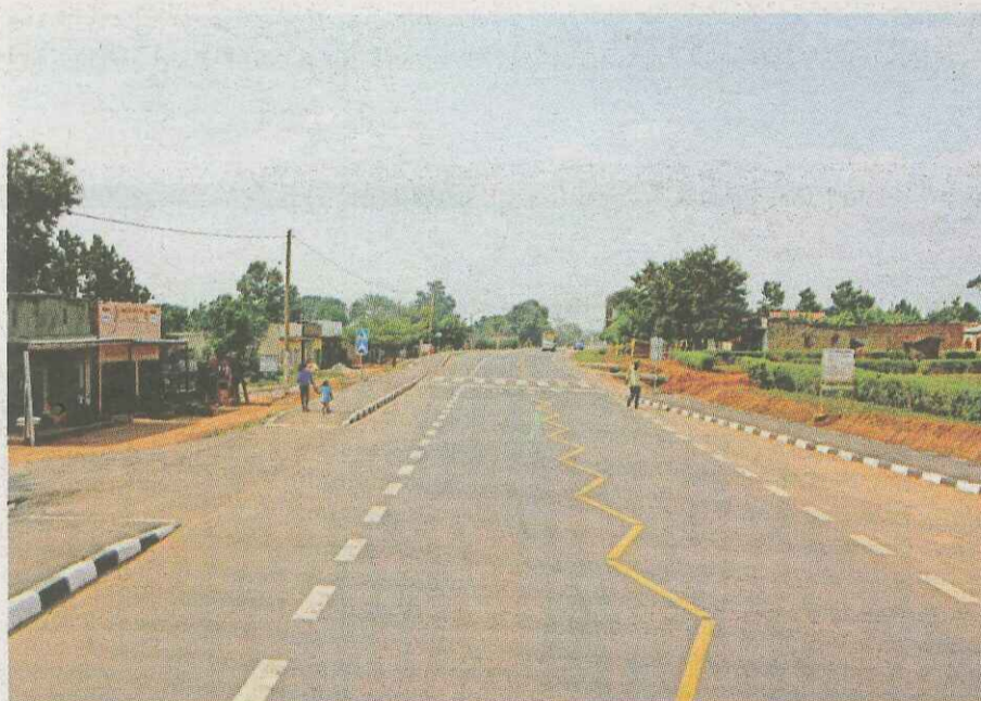
Completed. A section of the finished road in Kayunga District. COURTESY PHOTO
